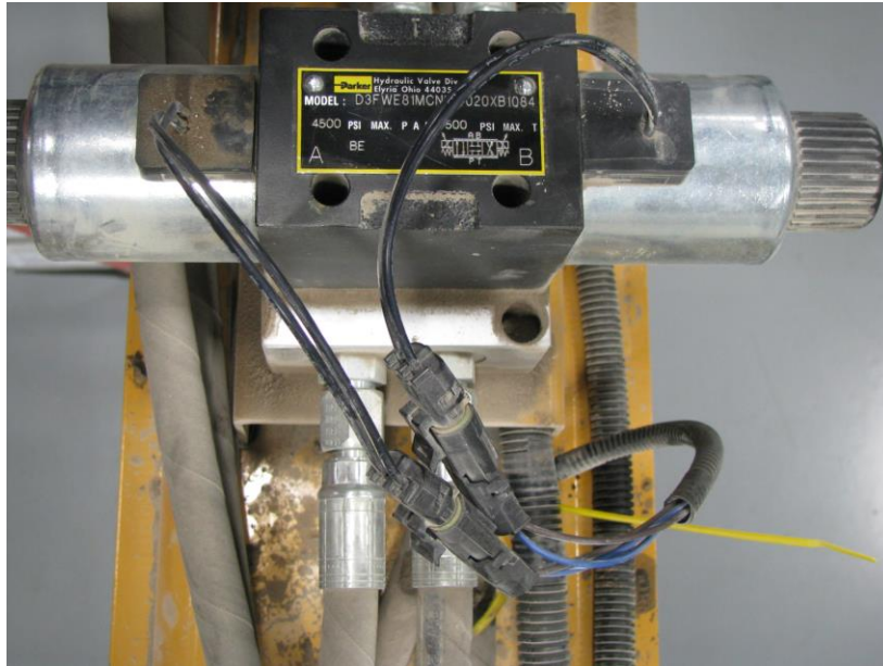
Figure 10. Proportional valve connections
